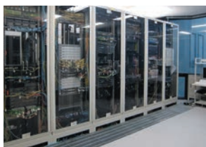
Network Operation Center
